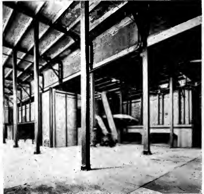
Showing back of furnace units with fan for forced draft. Draft is preheated by passing through a regenerator.
